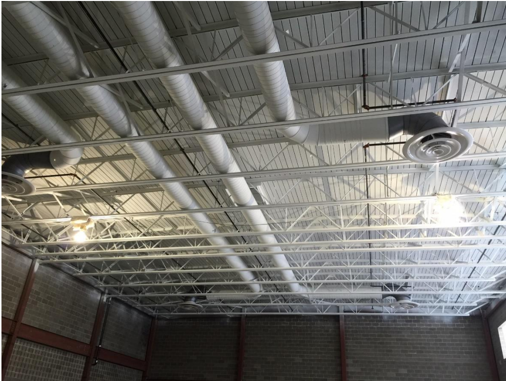
Sprinkler piping and duct work in gym
