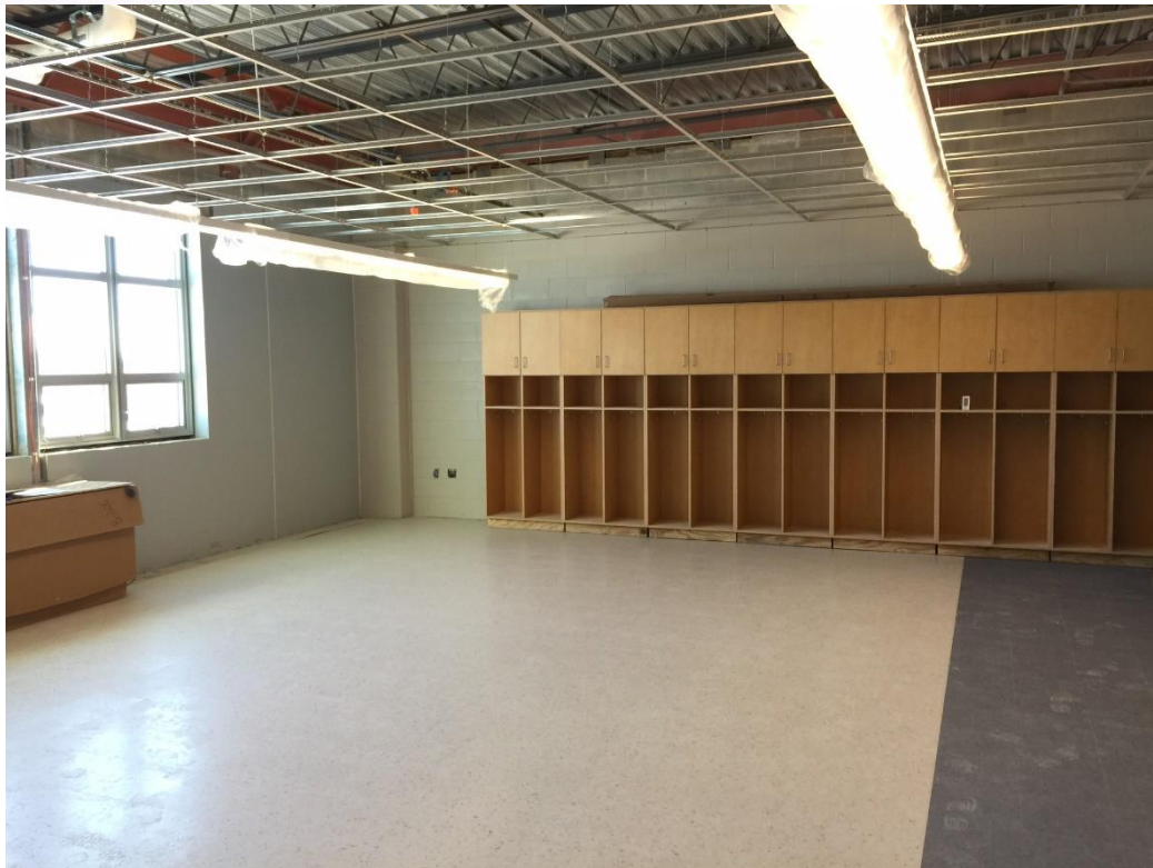
Classroom lights and VCT
